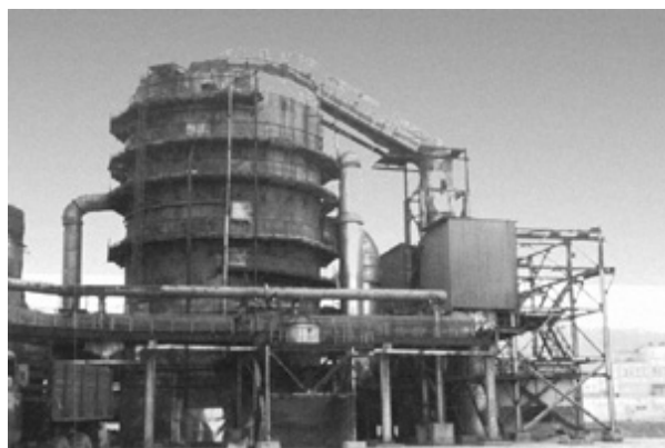
Fig. 13. Reverse-flow reactor for oxidation of SO 2 at Pechenga Nickel Smelter (Nickel town, Russia).
